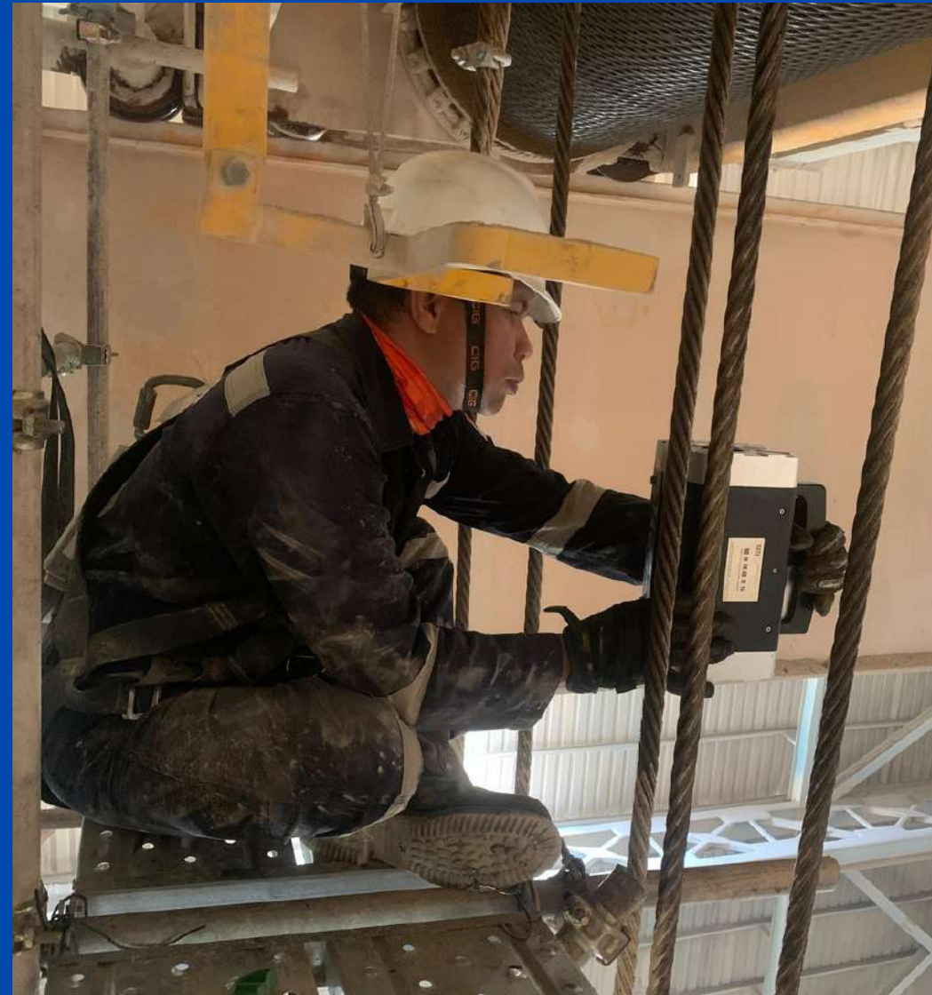
INDOCEMENT BOSOWA MAROS MAKASSAR Wire Rope Tester OHC 75 Tonnes Capacity
