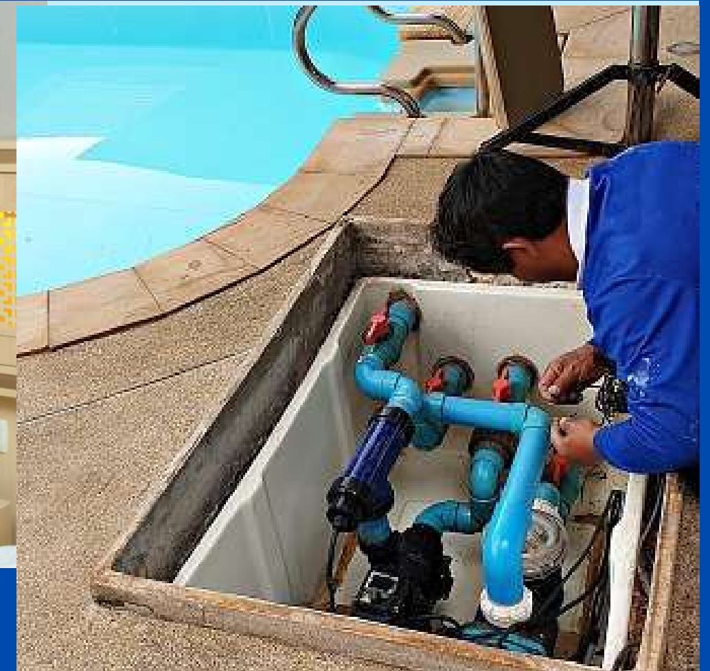
THE BLUE SKY HOTEL BALIKPAPAN Electrical Facility & Swimming Pool maintenance
